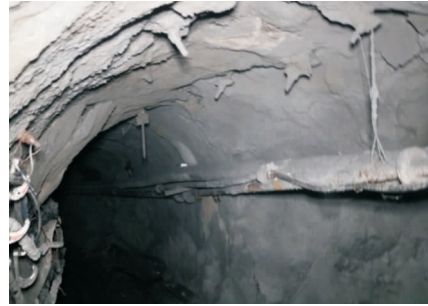
图5 返修后锚杆托盘与顶板严重分离
